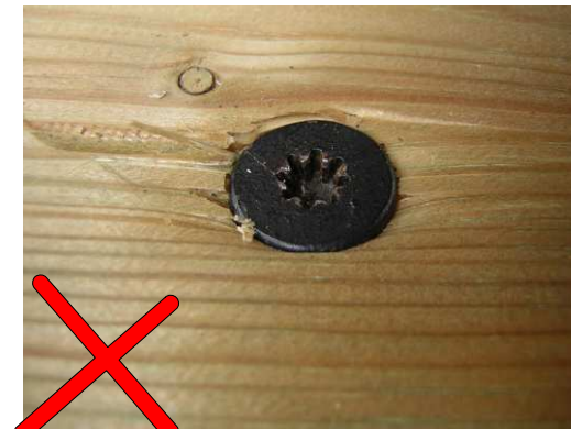
SPLITS & CRACKS AROUND SCREW HEAD
